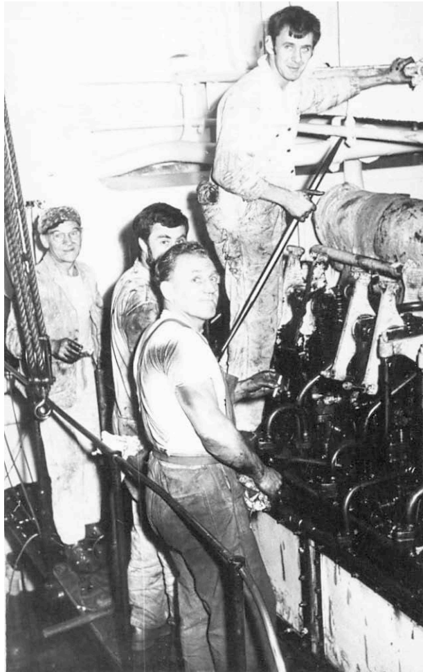
Generator Repairs Left to Right Donkey Man, Brian Hinchcliffe, Greaser, Barrie Hudd
